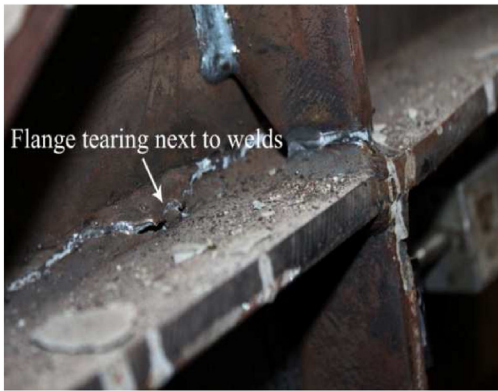
(e) Beam flange fracture in frame 1 on the first storey
