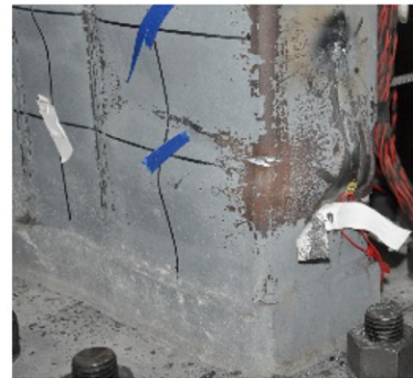
(b) Local buckling
