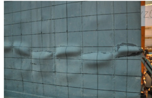
(b) Local buckling from the front view
