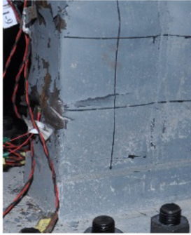
(b) Horizontal crack in the weld
