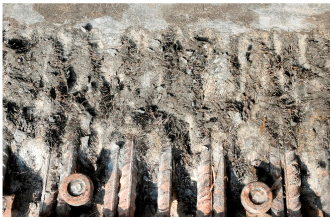
Fig. 7. Surface roughening after demolding
