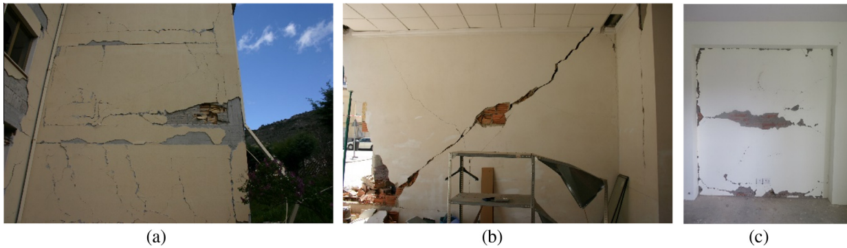
Fig. 1. Typical damage observed on in-plane IM walls: (a) detachment of the surrounding RC frame in the L'Aquila (Italy) earthquake, (b) diagonal cracking in Lorca (Spain) and (c) in the Nepal earthquake.
