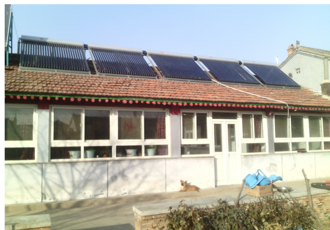
Fig. 1. The pilot household of the solar space heating system combined with a ASHP in the rural region of Beijing.
