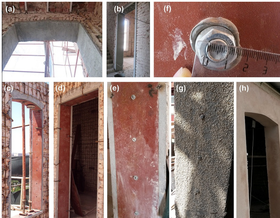
Fig. 9. Application of steel plate profiles on door and window gaps: (a and b) Composing a surface with polymer modified mortar with 3 cm thickness grout additive, (c–f) Steel plate assemble on door and window edge surfaces, (g) Preparing the surface for plaster application, (h) Plaster reproduction to conceal the steel plates.
