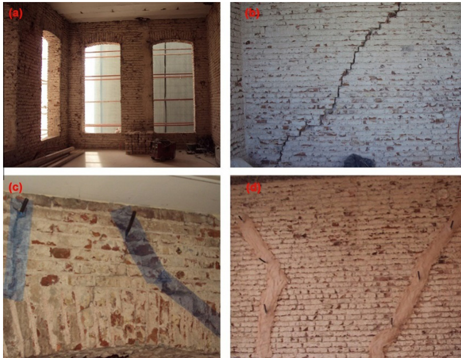
Fig. 7. Application of wall injection: (a) Examination of all the walls after the plaster removal, (b) Determination of structural cracks, (c) Preparation of the surface for injection, (d) Completing injection application with manual technique.
