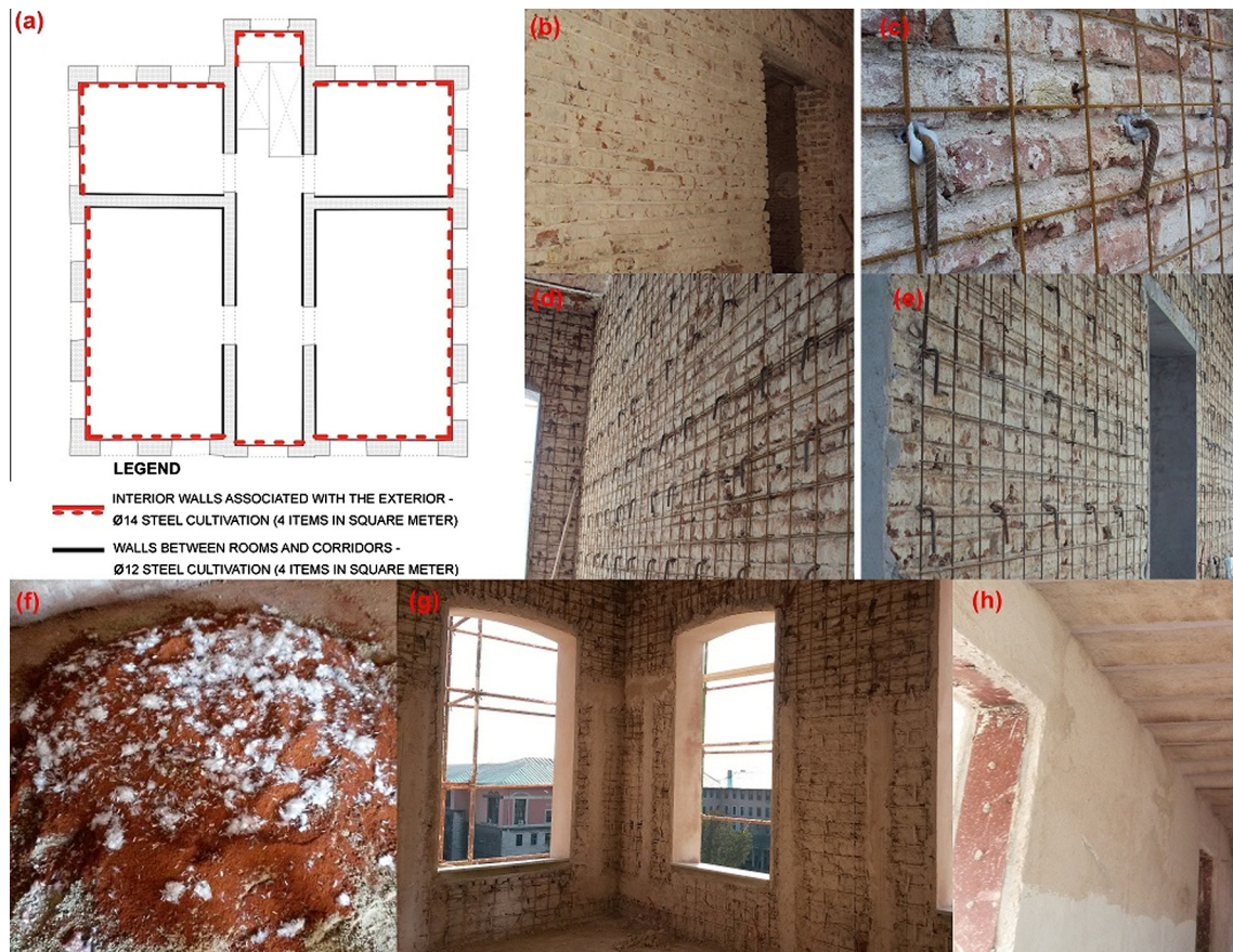
Fig. 12. Strengthening the internal walls with ore plantation method: (a) Strengthening locations of the first- and second-floor walls (interior), (b) View of the wall after plaster removal, (c–e) Strengthening the wall by using wire mesh, (f) Using polypropylene fibers in plaster content, (g) Application of thick plaster, (h) Application of thin plaster.
