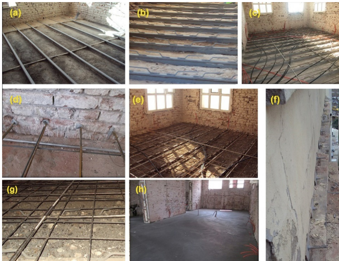
Fig. 8. Strengthening of the brick floor arches: (a) Removing top layers of the slab, adding \phi 10 shear rebar on the slab profile beam and painting with antirust paint, (b) Assembling shear rebars on the steel beams in the volta slabs, (c) Steel tie fabrication, (d) Planting the ores on the masonry walls, (e) Completing the welded wire fabrication, (f) Completion of the connections of stainless steel ties between the masonry walls, (g) Stretching the stainless steel profiles, (h) Topping concrete application on the slab.
