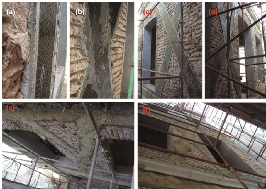
Fig. 11. Exterior facade application of carbon fiber wrap: (a and b) Detail of polymer modified mortar with 3 cm thickness, (c–f) Preparation by spraying quartz sand to make it ready for plaster.
