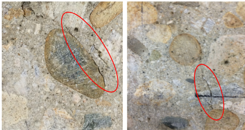
(b) Cracks on surface (60% of compressive loading)
