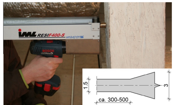
Fig. 3. Resistance drilling device during timber column testing. Drill shape and dimensions (mm) are shown in lower right corner.
