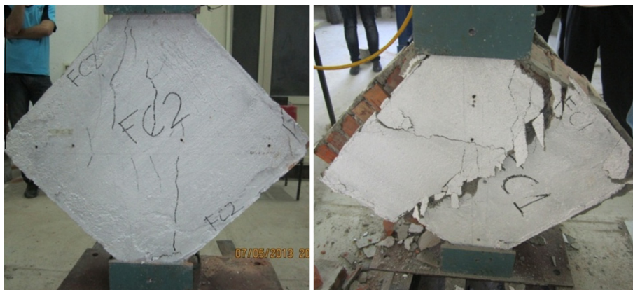
Fig. 7. Ferrocement jacketed wall: (a) hair-like cracks developing along the compressed diagonal; (b) yield of the jacket and total failure of second specimen.
