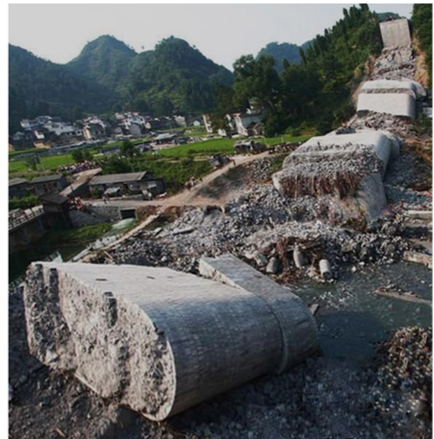
Fig. 4. Collapse scene of Tuojiang Bridge (image courtesy of Long Xiao)
