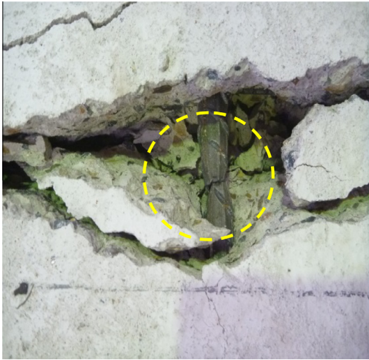
Fig. 11. Typical failure mode of the specimens associated with rupture of reinforcing bars.
