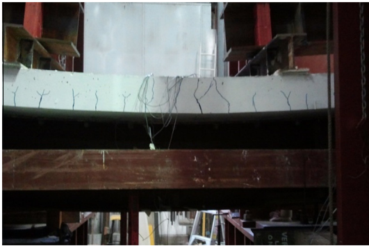
Fig. 16. Vertical concrete cracks on bottom and side faces of concrete slab.
