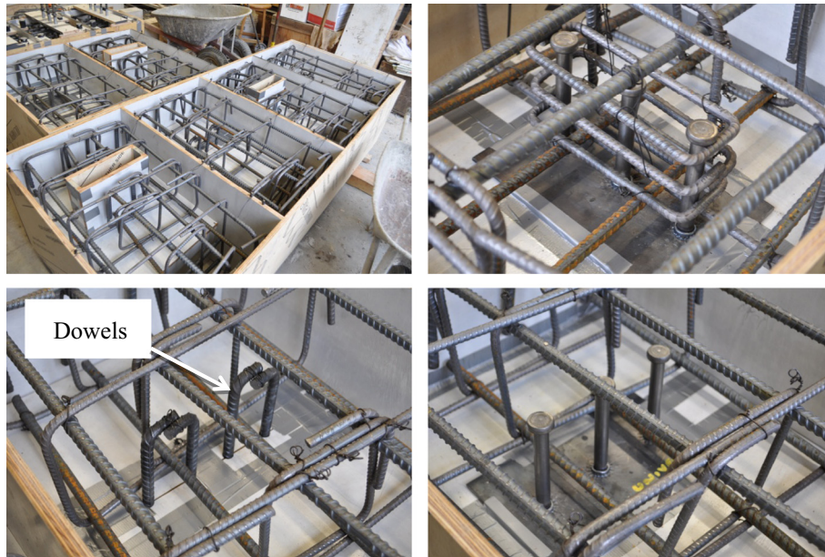
Fig. 3. Clockwise from top left: (a) reinforcing cages and formwork, (b) confined studs, (c) unconfined studs and (d) rebar dowels.
