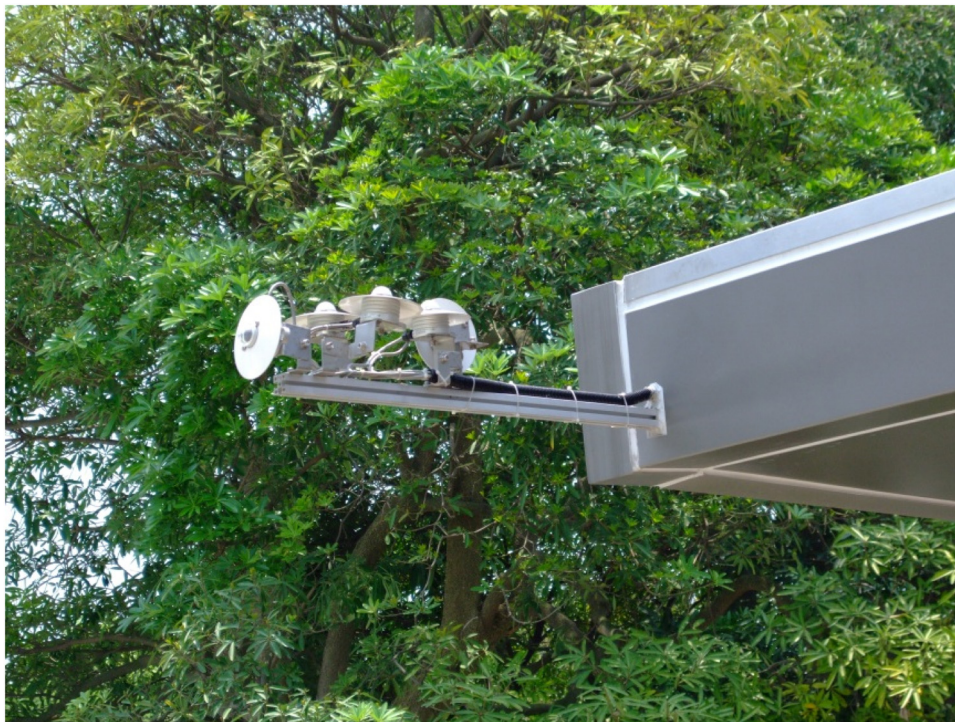
Fig. 4. The pyranometers of the BIPV Experiment Demonstration House.
