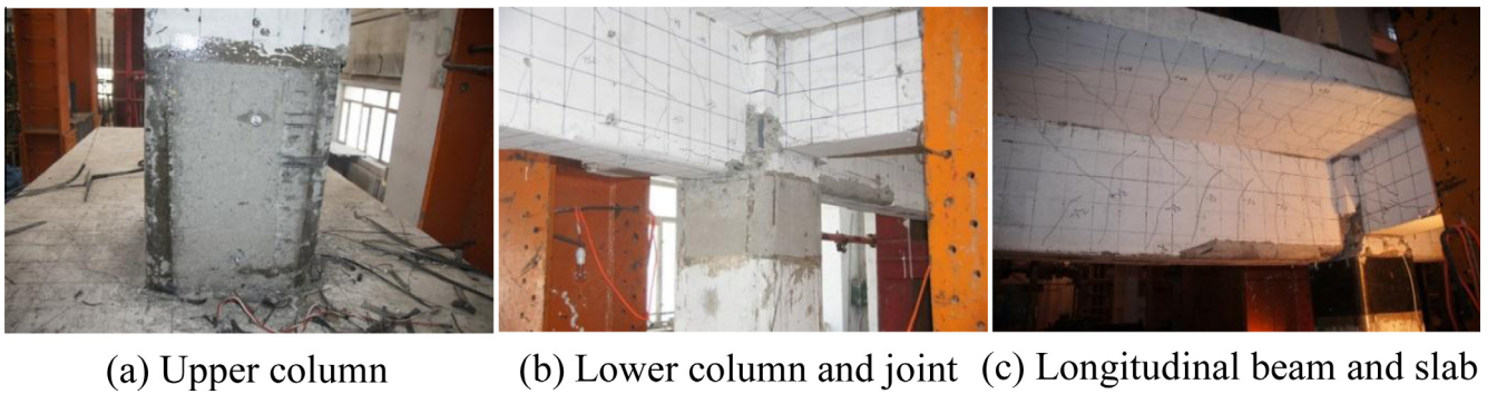
Fig. 8. Failure modes of specimen SC.
