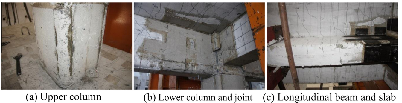
Fig. 9. Failure modes of specimen SCBU.
